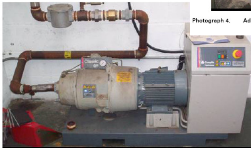
Photograph 3. Gas compressor model HV07
